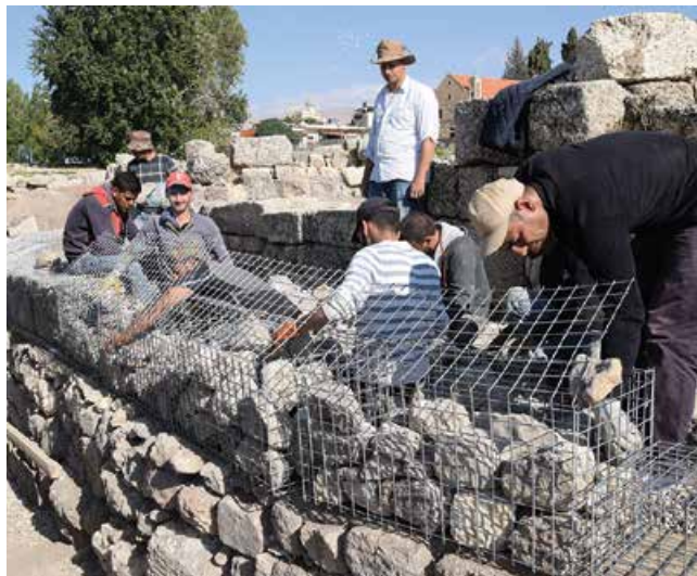
Fig. 11: Baalbek, Bustan Nassif. Gabion walls were built where larger protection structures were needed (Photo: DAI, Julia Nádor)
