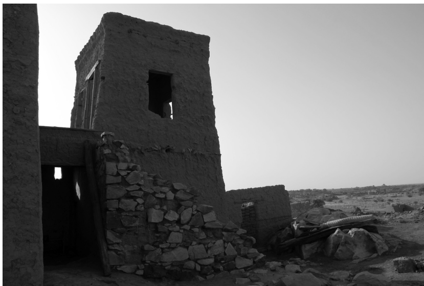
Fig. 12: The curated and partially restored 'tower' in Malik al-Farah's compound (photo: C. Kleinitz)
