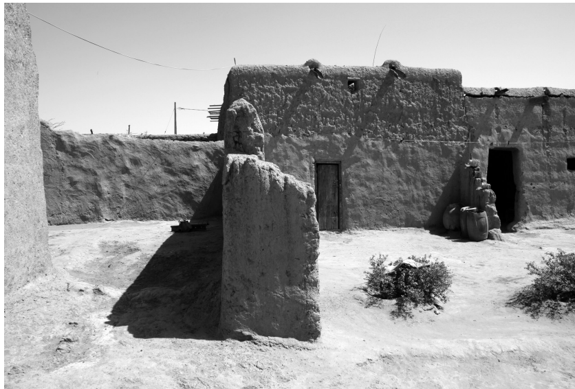
Fig. 9: Multiple episodes of building and modification are visible in the mudbrick fabric of the Basheere family's compound (photo: C. Kleinitz)
