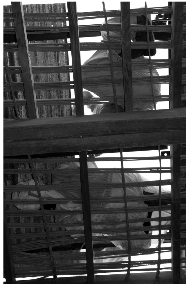
Fig. 3: Preparing the roof of the Lion Temple for investigation, October 2014 (photo: Claudia Näser)
