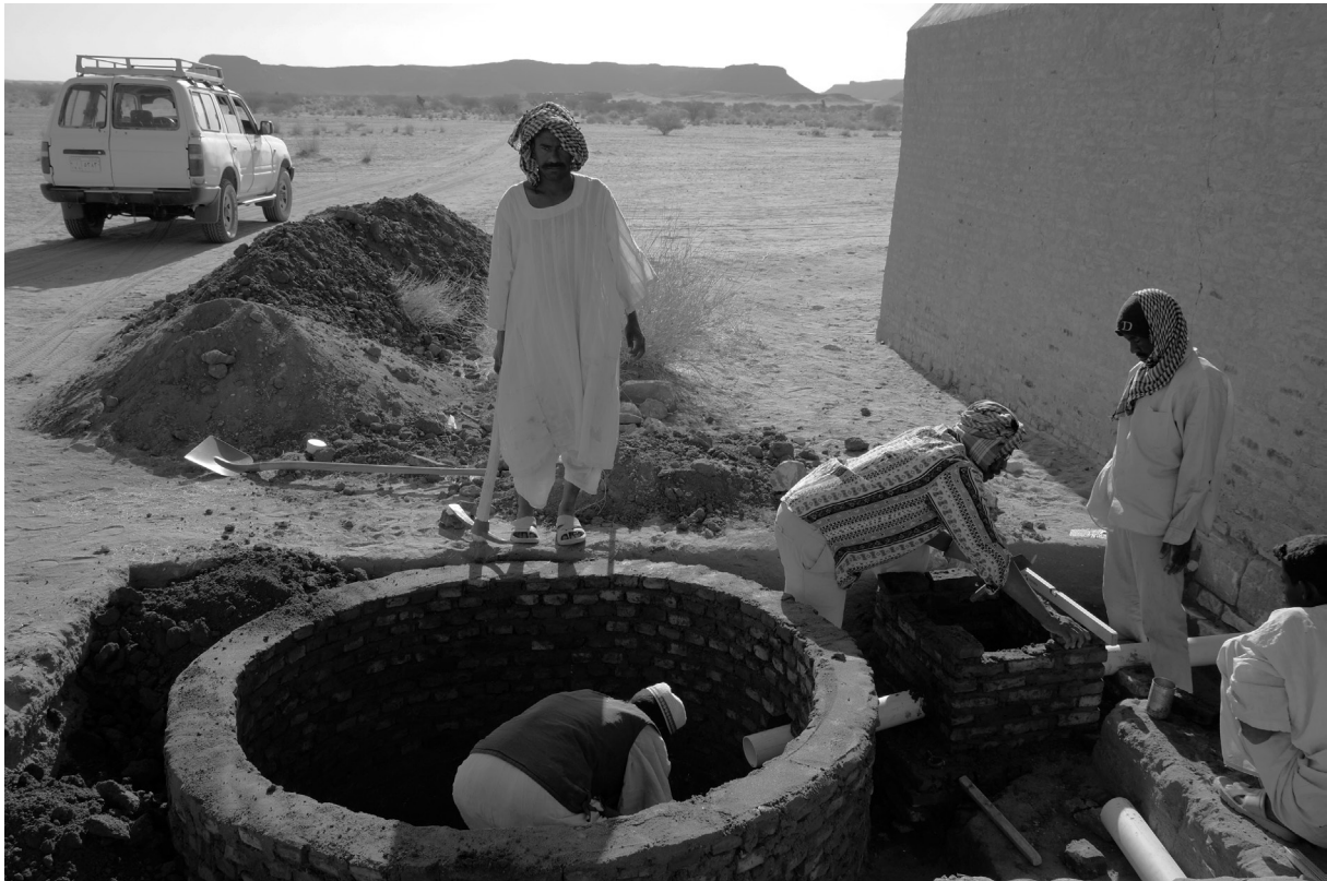
Fig. 20: Construction of the infiltration well outside the enclosure wall (photo: Claudia Näser)
