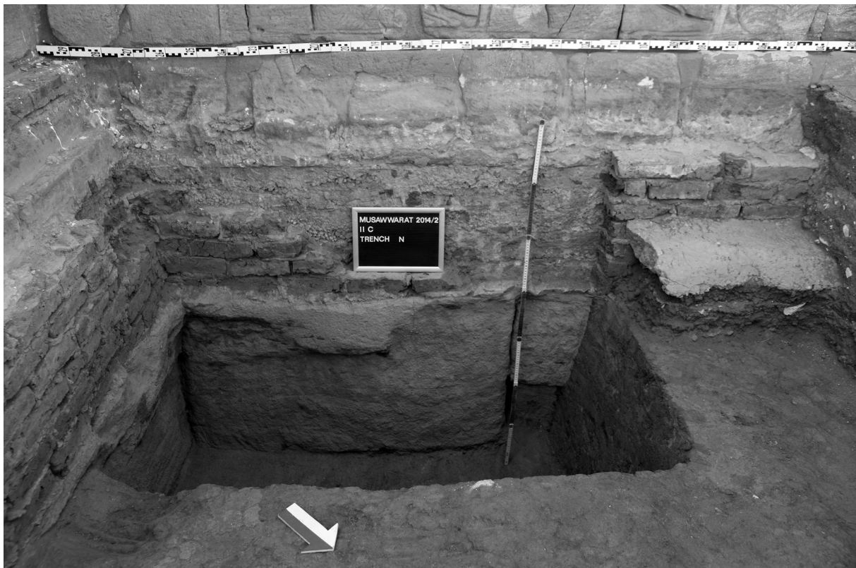
Fig. 5: The foundations of the reconstructed Lion Temple consisting of a mighty unreinforced concrete body underneath the actual reinforced concrete foundations, the brick-lining of which has been supported by a concrete ‘shirt’ (preserved on the right side), exposed in the trench in the rear of the northern pylon tower (photo: Claudia Näser)
