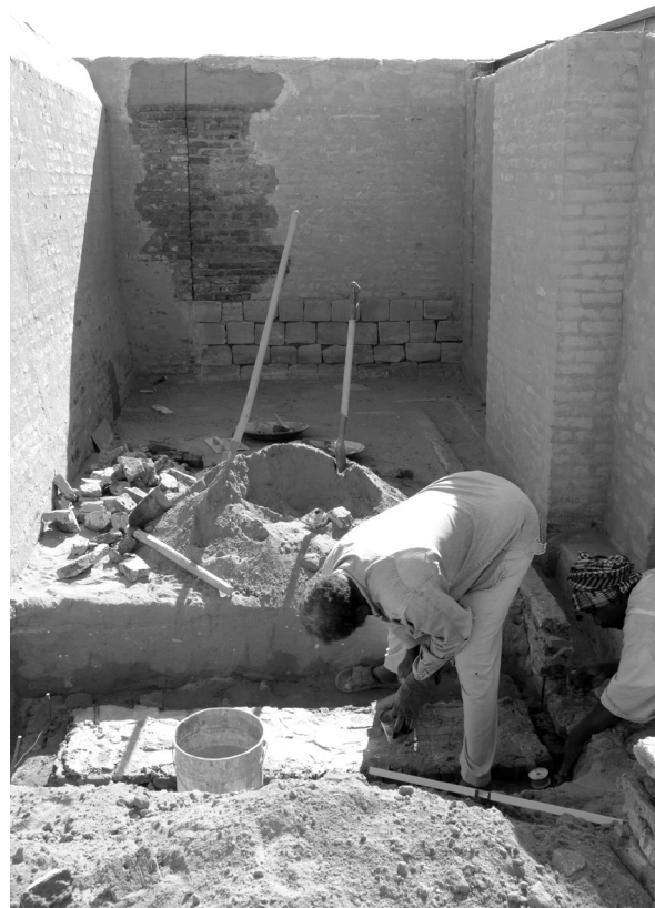
Fig. 19: Construction of the new outlet channel for the drainage of the site museum; note the re-modeled, though still unplastered area of the crack in the enclosure wall in the rear (photo: Claudia Näser)
