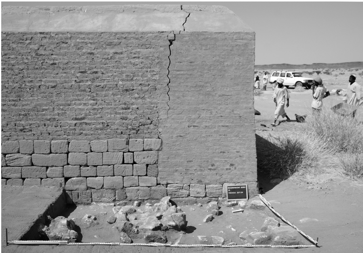
Fig. 18: Crack in the reconstructed enclosure wall at the northeastern corner of the Great Enclosure (photo: Claudia Näser)
