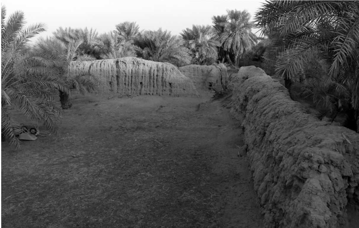
Fig. 5: The southeastern and northwestern walls of al-Hilla fortress, facing northwest (photo: Gareth Rees)
