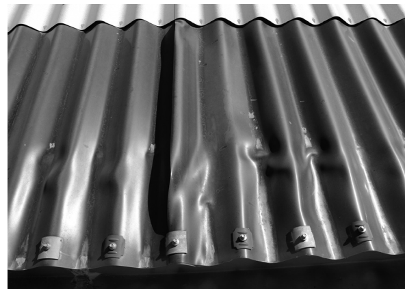
Fig. 8: Deformed PVC sheets on the Apedemak Temple's roof (photo: Cornelia Kleinitz).
