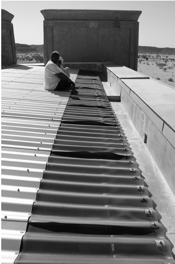
Fig. 7: Deformed PVC sheets from the light slits along the sides of the Apedemak Temple's roof (photo: Cornelia Kleinitz).
