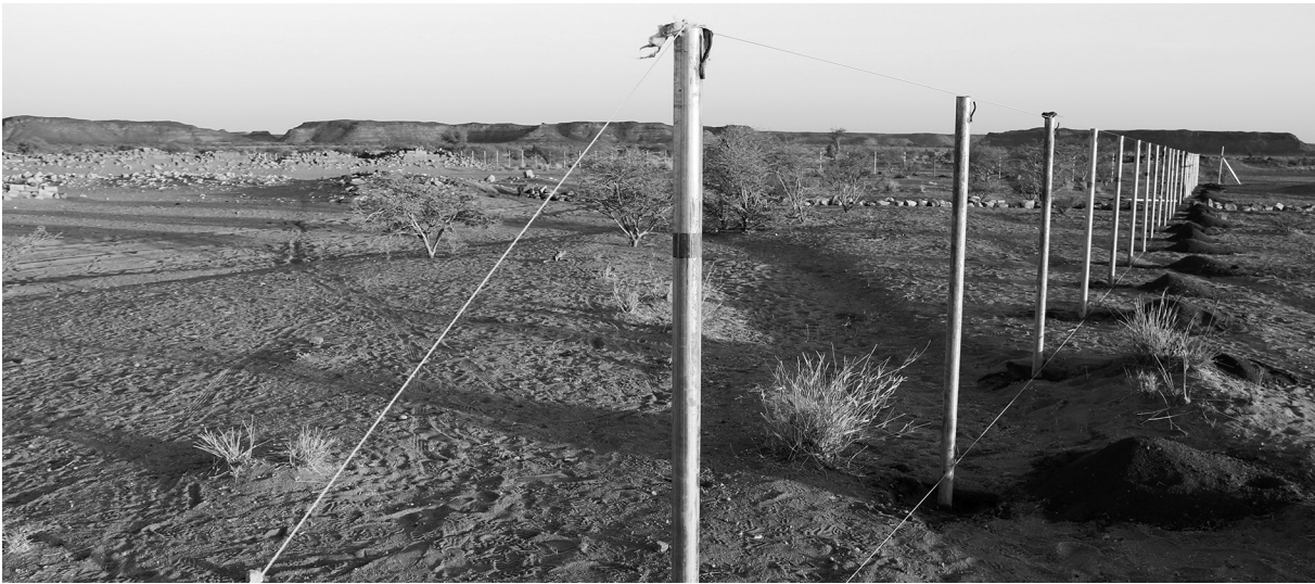
Fig. 31: Metal poles on the western side of the Great Enclosure during the construction of the perimeter fence (photo: Cornelia Kleinitz).
