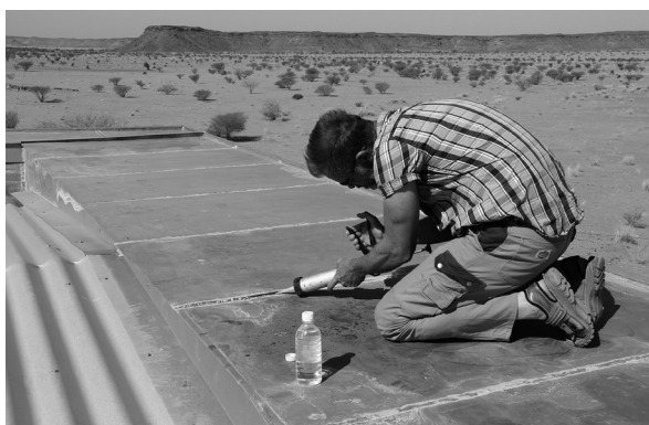
Fig. 10: Provisional repairs to the seams between the zinc sheets of the parapet of the Apedemak Temple's roof (photo: Cornelia Kleinitz).
