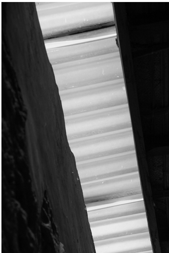
Fig. 9: Loss of translucency in the PVC sheets from the light slits of the Apedemak Temple's roof (photo: Cornelia Kleinitz).
