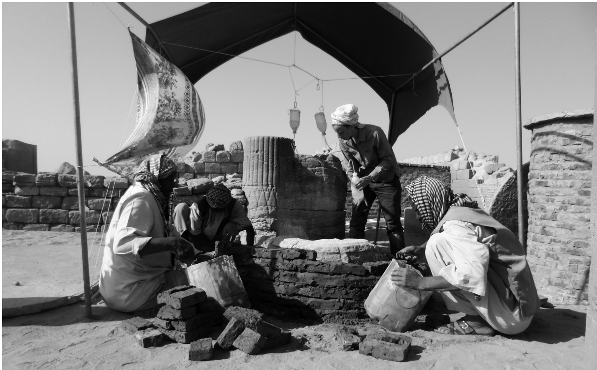
Fig. 24: Conservation of column 5 in progress: Infusion and flooding of column drums with colloidal silica solution (photo: Alfatih Mohamed Ali Saeed).
