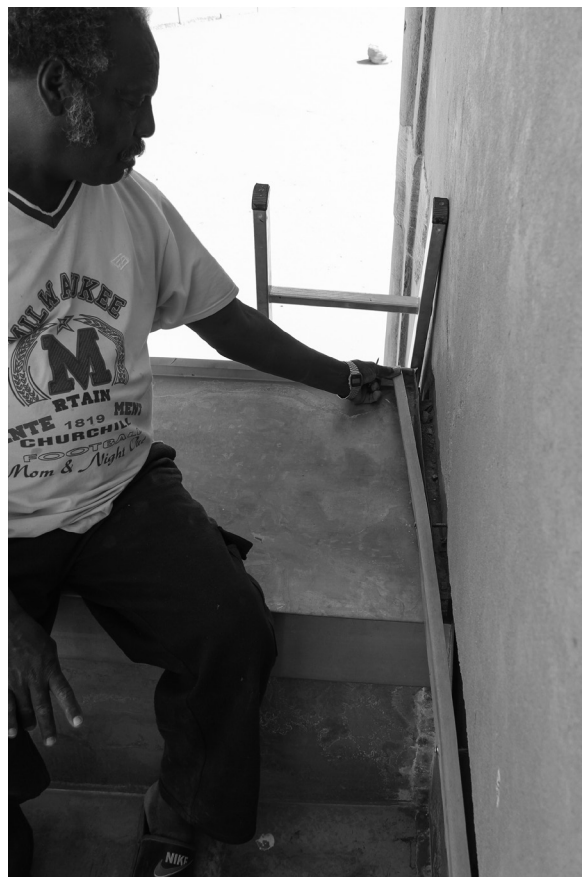
Fig. 11: Loose connection between zinc sheets of the roof and pylon of the Apedemak Temple (photo: Cornelia Kleinitz).
