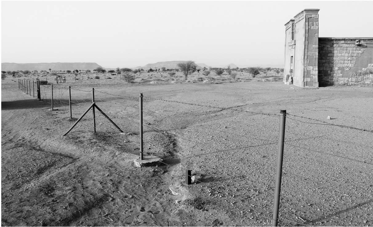
Fig. 34: Erosion gullies in the vicinity of the Apedemak Temple (photo: Cornelia Kleinitz).
