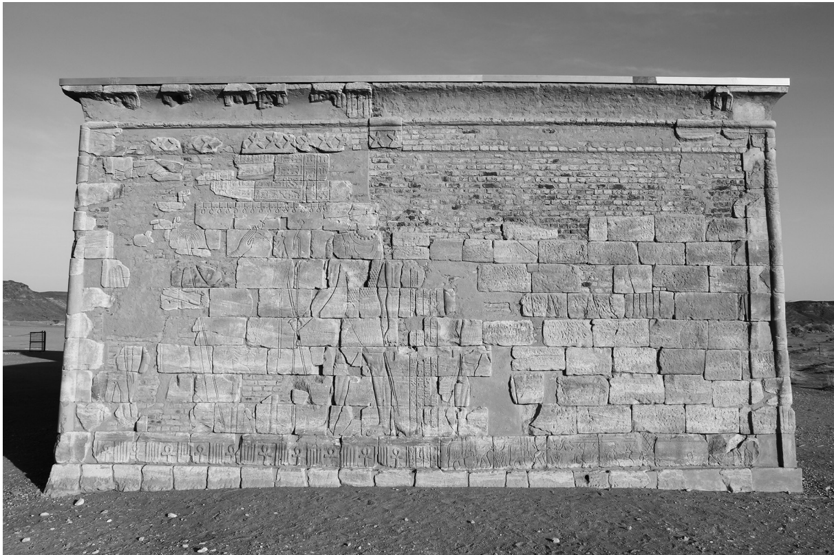
Fig. 6: Section of missing plaster on the outer west wall of the Apedemak Temple (photo: Cornelia Kleinitz).
