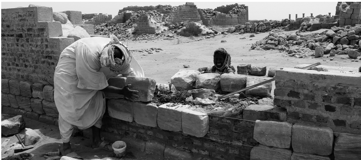
Fig. 29: Increasing the height of a section of the northern enclosure wall of the Great Enclosure (photo: Cornelia Kleinitz).
