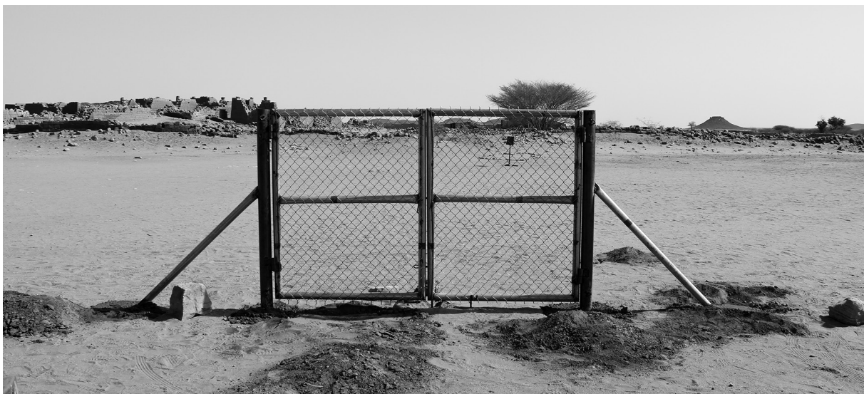
Fig. 30: Main (visitor) gate of the fence for the Great Enclosure immediately after installation (photo: Cornelia Kleinitz).
