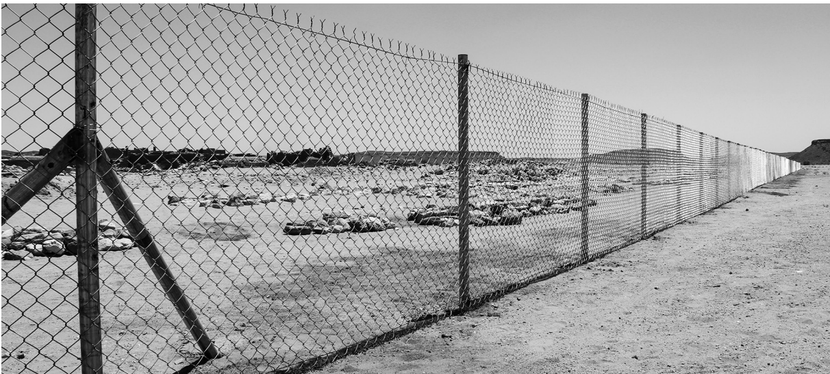
Fig. 32: Western side of the fence of the Great Enclosure after the completion of work (photo: Cornelia Kleinitz).
