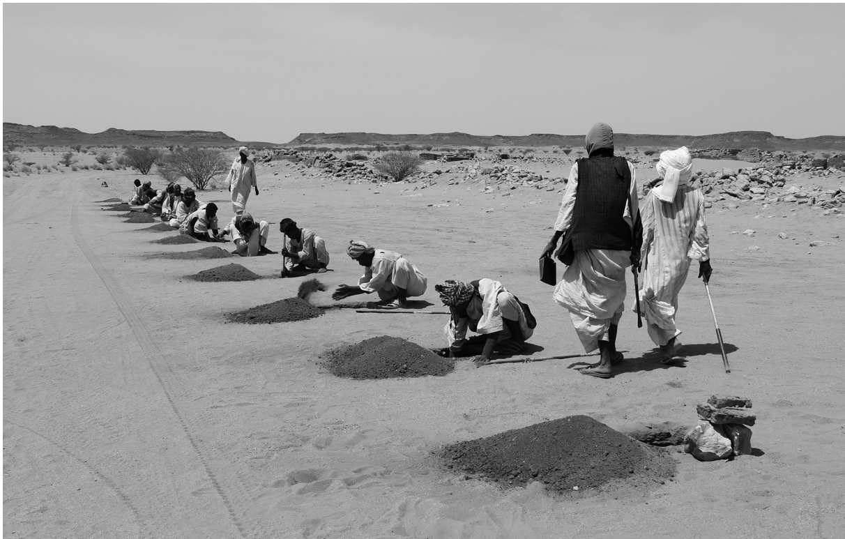
Fig. 27: Digging the foundation pits for the poles of the fence to the south of the Great Enclosure (photo: Cornelia Kleinitz).
