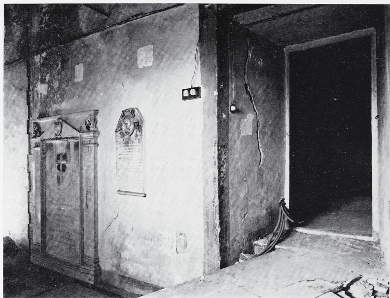
17 The eastern wall of Room A. This wall was originally an exterior wall.
