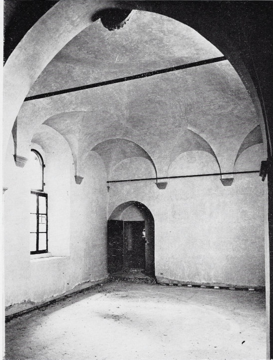
6 Room B viewed from its chapel. This room was originally the Busini sacristy.
