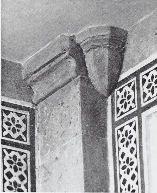
9 Detail of one of the pilasters and consoles in Room A (see Fig. 2: no. 3).
