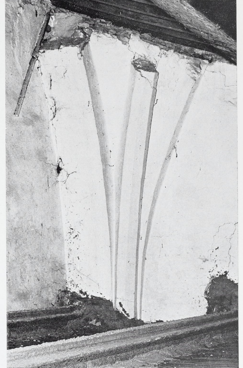
10 Detail of the rib and arch above the present ceiling of Room A. The ceiling is modern and these formed part of the original vault of Room A.
