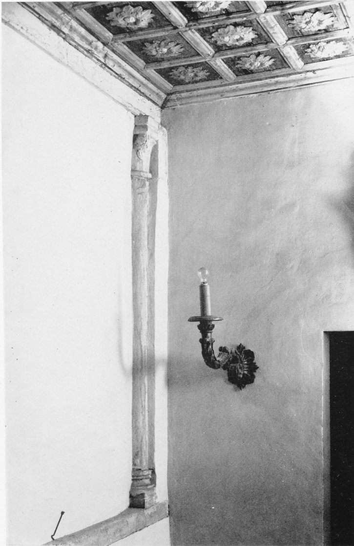
32 Colonnette in the south-west corner of the loggia on the piano nobile .
