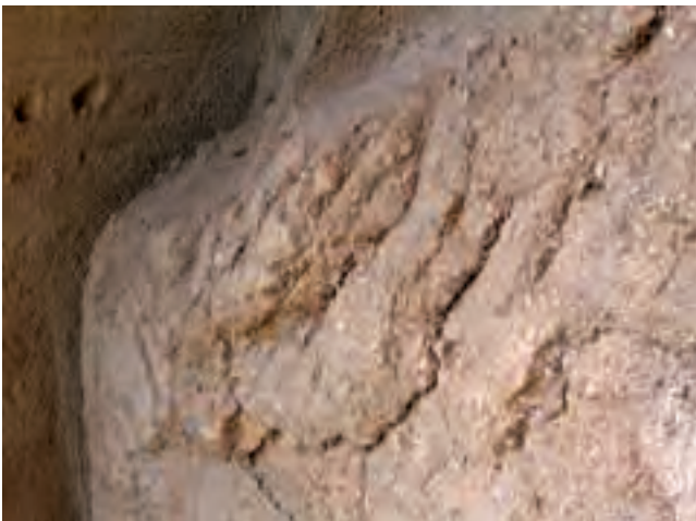
Fig. 19. Right shoulder of the Small Buddha (new discontinuities parallel to the back wall)
