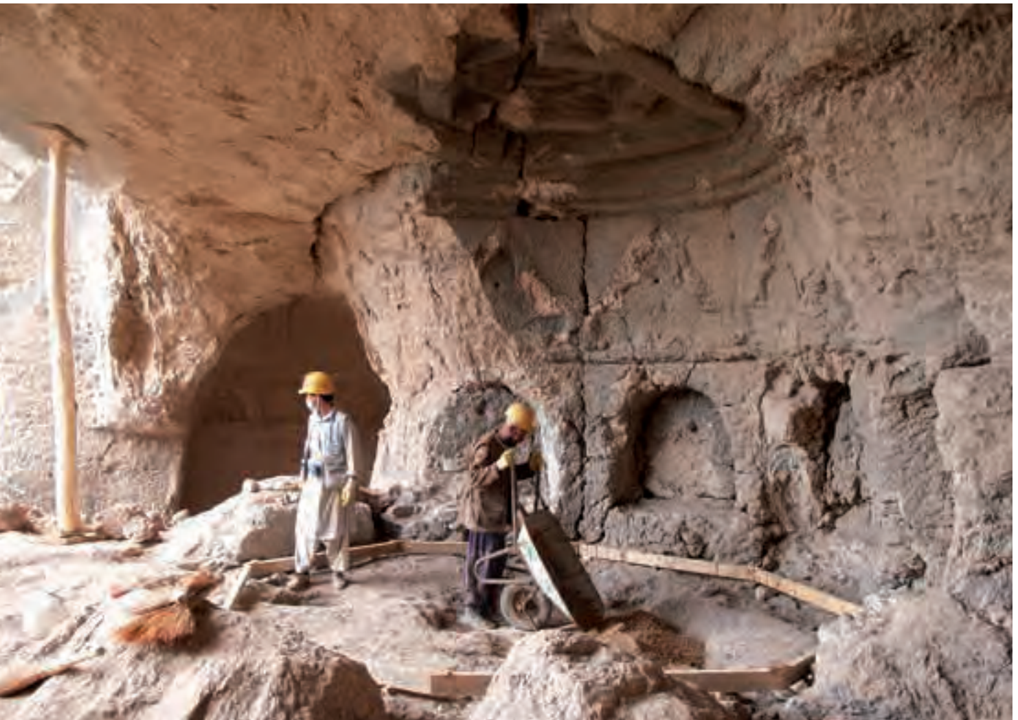
Preparing the reconstruction of the partition walls in the niche of the Eastern Buddha
