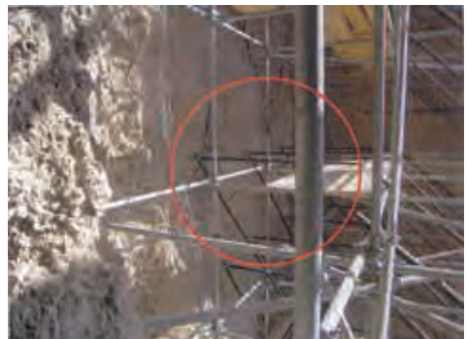
Fig. 1. Extensions made to the original scaffold consist of two grounded towers to a maximum height of about 20 meters above ground. Shown here is balcony type in the upper part. Any extensions to the scaffold reaching up higher were avoided in order to not interfere with the most unstable parts of the rock surface within and directly below the shoulder area.
