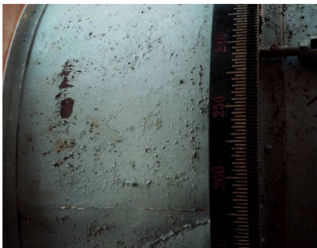
Figure 32.2: Lac flaking off and corrosion are the main problems of instruments in observatory (HTW, Keller-Kempas)
