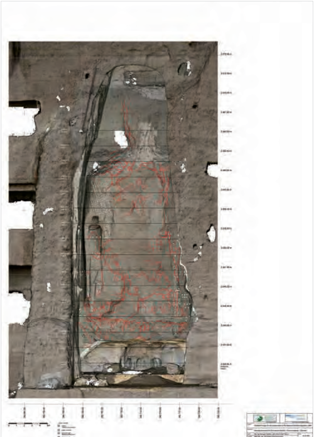
Fig. 9. Eastern Buddha niche, damage assessment of the back wall
