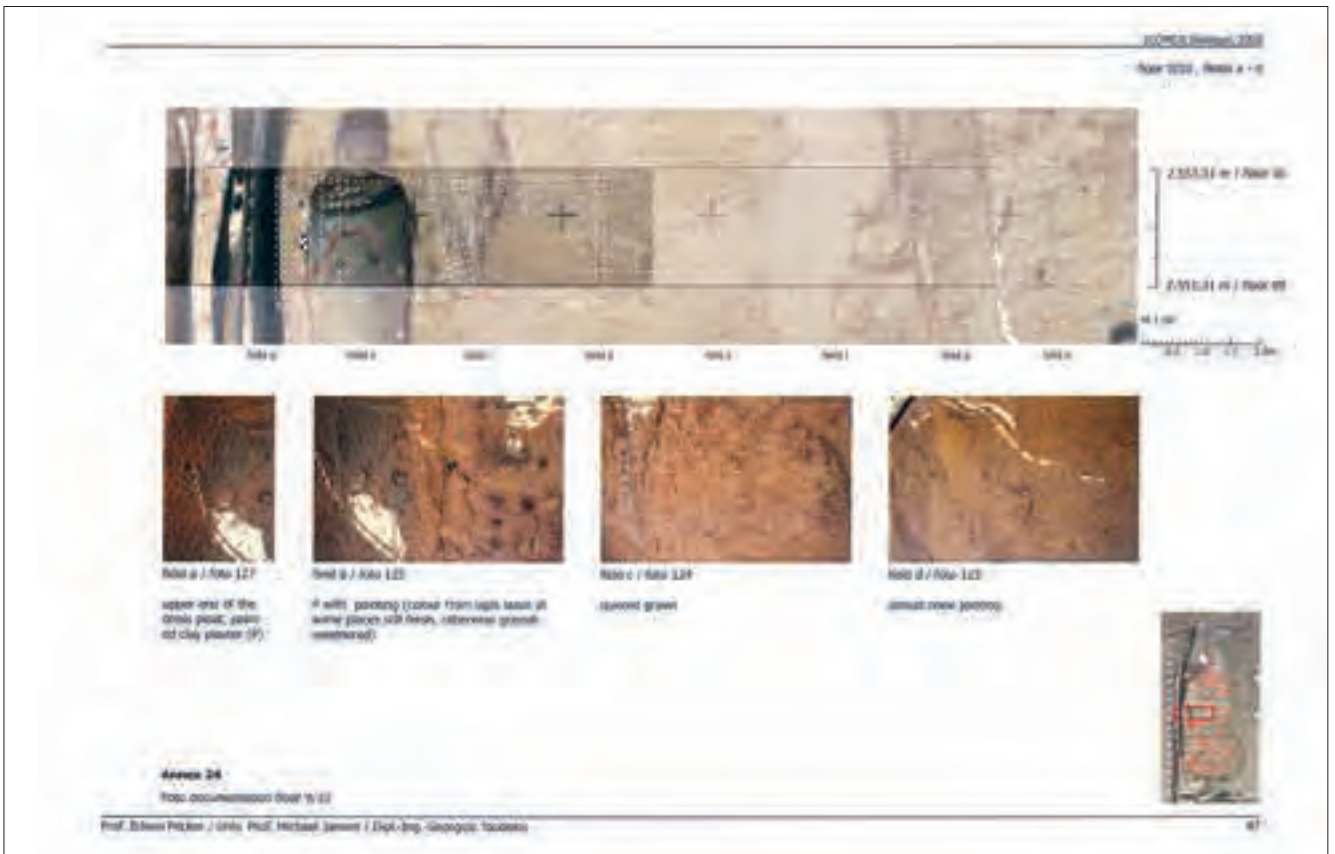
Fig. 14. Eastern Buddha, damage assessment, photo documentation, floor 9/10
