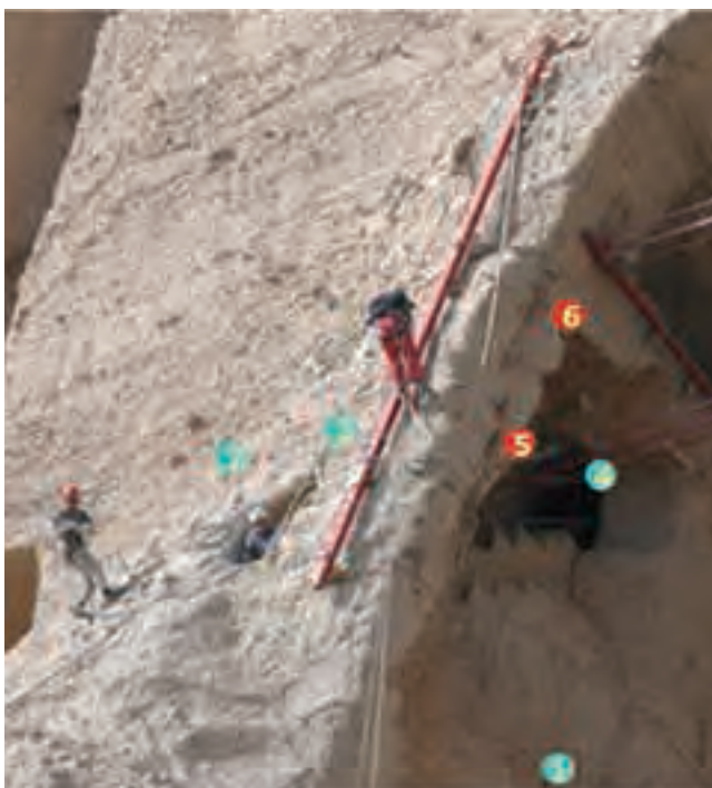
Fig. 26. The location of potentiometric crack gauges for discontinuity monitoring and alarm; in green are external sensors and red are internal to the cave
