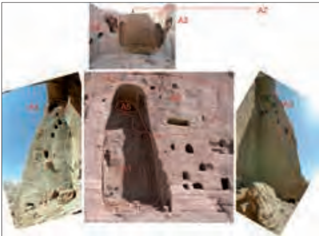
Fig. 8. Identification of the most critical instability areas in the Eastern Giant Buddha niche. The A3 block in the Eastern Giant Buddha niche exhibits the most acute instability
