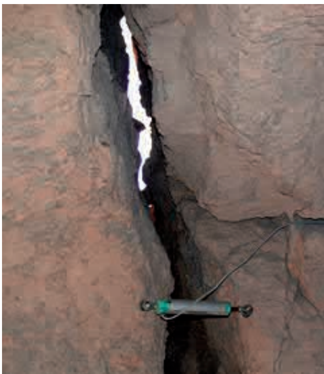
▽ Fig. 12. Distribution of the 11 sensors monitoring the crack's underlining of the most unstable block. On the left a detail of such sensors
