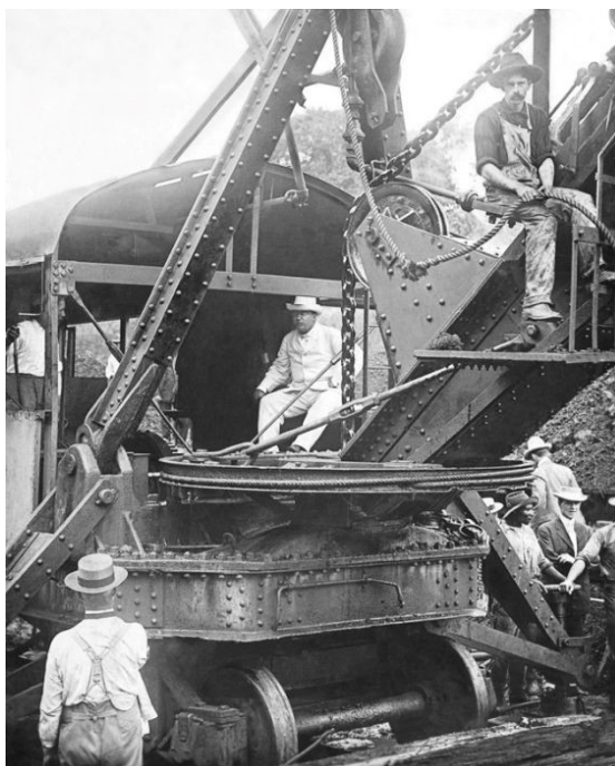
1 President Theodore Roosevelt in the cab of a Bucyrus shovel at the Culebra Cut, Panama Canal, November 16, 1906. Library of Congress, Washington, D.C., Prints and Photographs Division (photo: https://www.loc.gov/item/2010649455/ )
