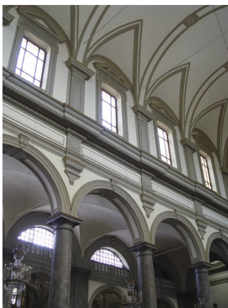
24 The church of San Domenico , Palermo, view of the aisles merging into the terraces above the side chapels (photo: K. Horvat-Levaj)
