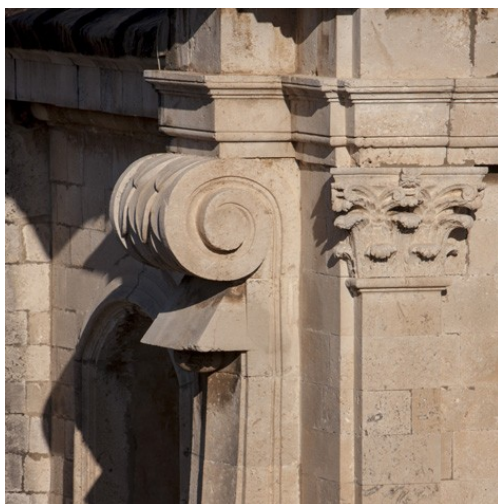
18 The Cathedral, Dubrovnik, buttresses from the vaulting of the main nave made according to the design by Tommaso Napoli (photo: P. Mofardin)
