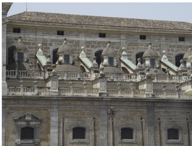
23 The church of San Giuseppe dei Theatini , Palermo, view of the terraces above the side chapels (photo: K. Horvat-Levaj)
