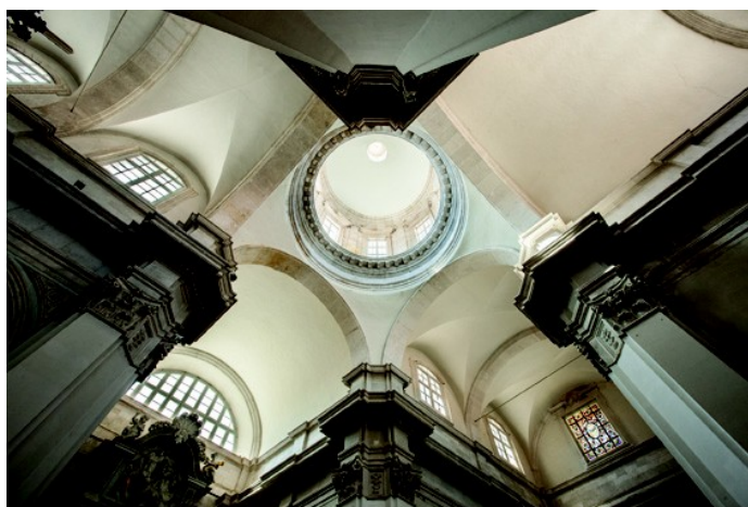
20 The Cathedral, Dubrovnik, cross vaulting in the nave and sanctuary made according to the design by Tommaso Napoli, and the barrel vaulting in the transept made in the time of Ilija Katičić according to the design of Andrea Bufalini (photo: P. Mofardin)
