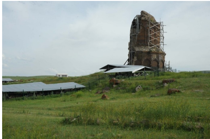
11 Church of Surb Prkich, Ani, general view of the site with the scaffolding and the shelters, June 2015 (photograph provided by A. Kazaryan)
