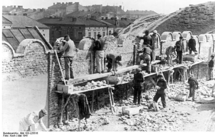
4 Construction of a wall for the Ghetto in the Podgórze district of Cracow, 1941, photo: Koch. Bundesarchiv, Koblenz, image 183-L25516
