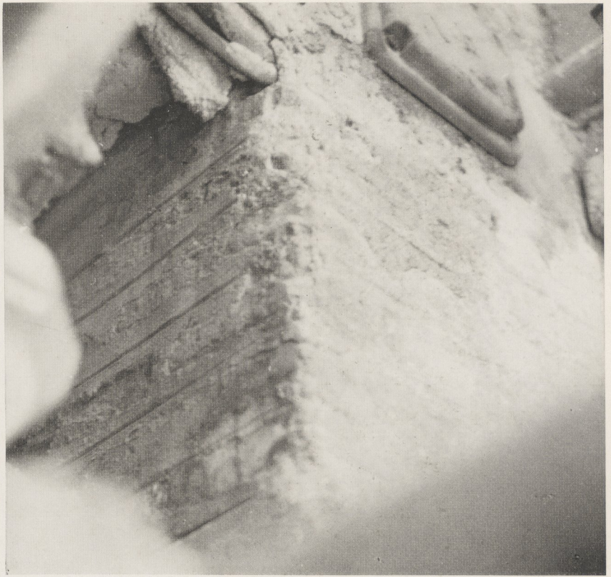
13. S. Maria in Aracoeli, falsa cortina on the west face of the early north-south wall
