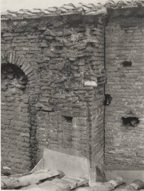
9. S. Maria in Aracoeli, southern arch opening in the west face of the campanile
